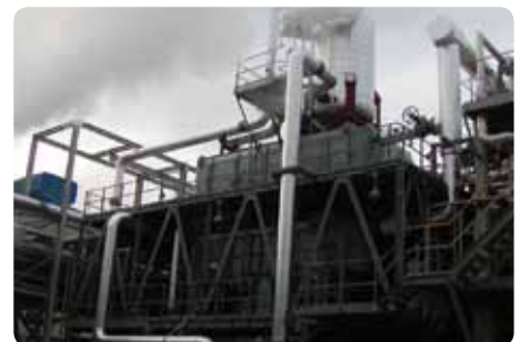
• 10 ton/h Absorption Heat Pump Installation [Korea]
